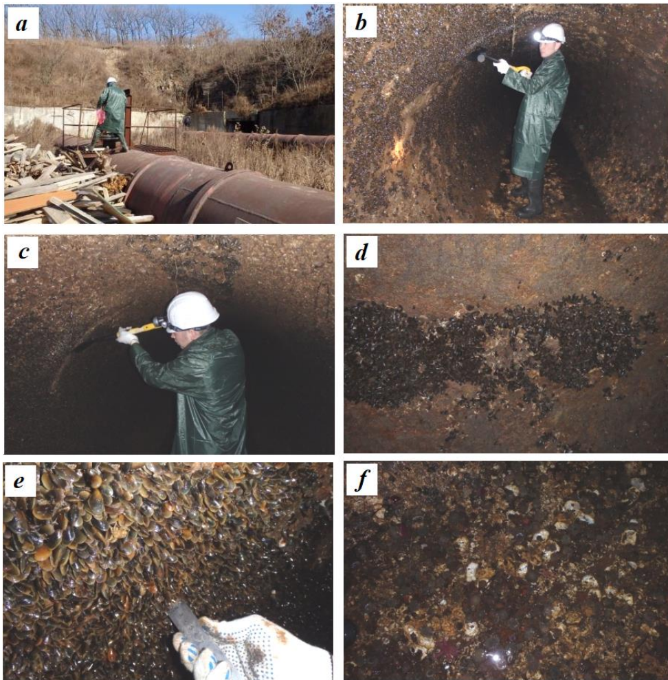
Fig. 2. The sampling process and general view of fouling of the water intake tunnel of CHP-2 in its different sections: a – beginning of the tunnel inspection, b – fouling by sessile polychaete worms of the genus Hydroides , c – test cleaning of the wall to assess the fouling intensity, d – mussel fouling, e – continuous mussel fouling of the tunnel, f – oyster fouling on the tunnel bottom
